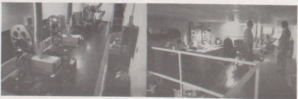
Fully automated projection rooms, each servicing two cinemas, are separated by upper level work area (pictured right).
